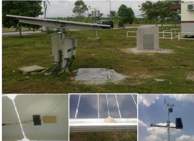
Figure 1: System setup for FF PV array with environmental sensors
